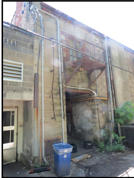
Image 12: North Elevation showing Door Opening and Balcony, 1014 King Street West, Hamilton – Westdale Theatre (Photo taken on May 29, 2017; Facing Southwest)
