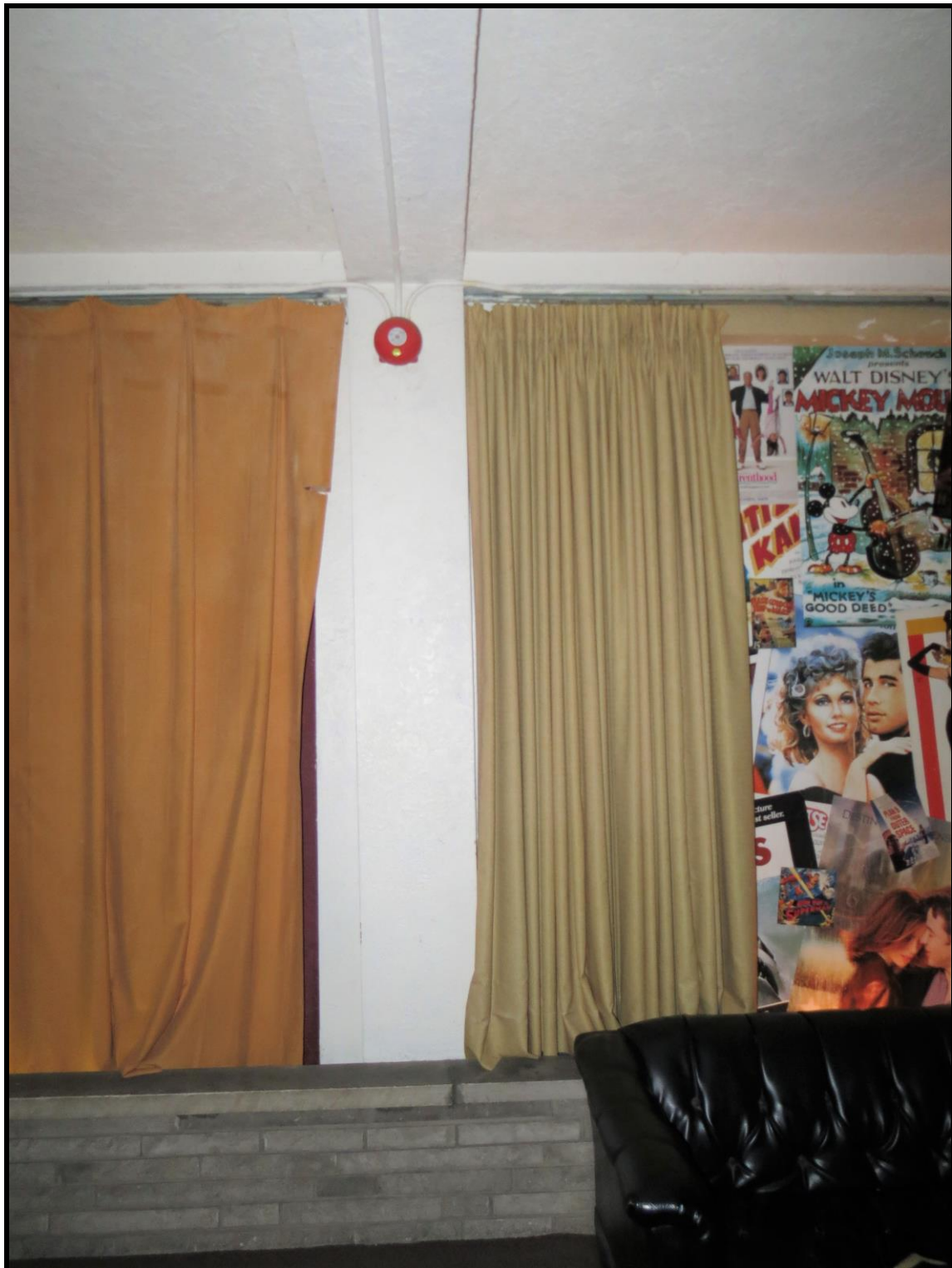
Image 34: Detail of Column on East Wall in the Foyer of 1014 King Street West, Hamilton – Westdale Theatre (Photo taken on May 29, 2017; Facing East)
