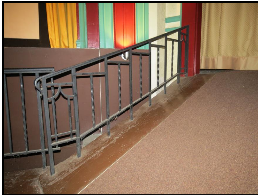
Image 42: Detail of Metal Railing on the Stage Ramp of 1014 King Street West, Hamilton – Westdale Theatre (Photo taken on May 29, 2017; Facing Northwest)
