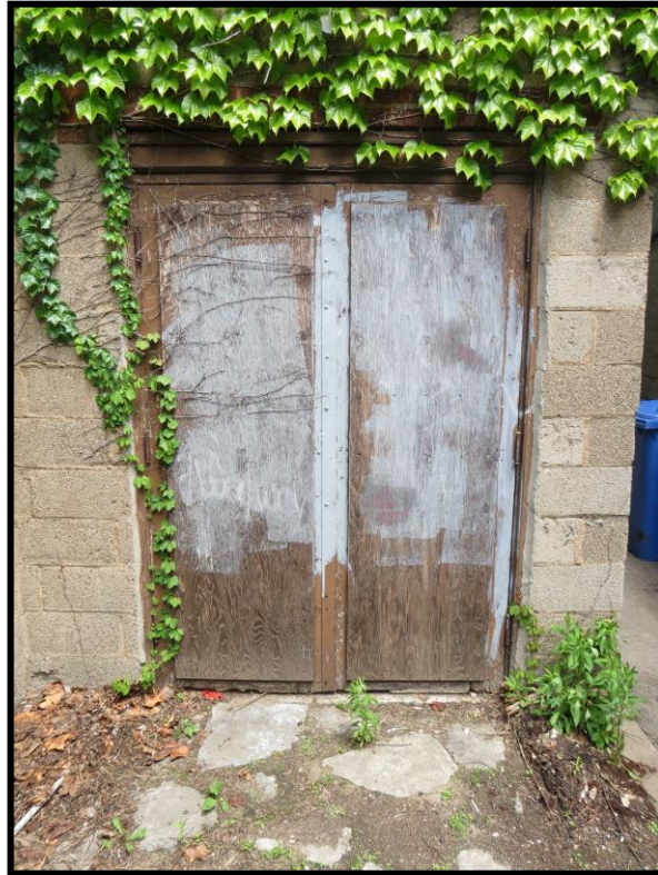
Image 10: Detail of Door Opening on Southwest side of West Elevation, 1014 King Street West, Hamilton – Westdale Theatre (Photo taken on May 29, 2017; Facing East)
