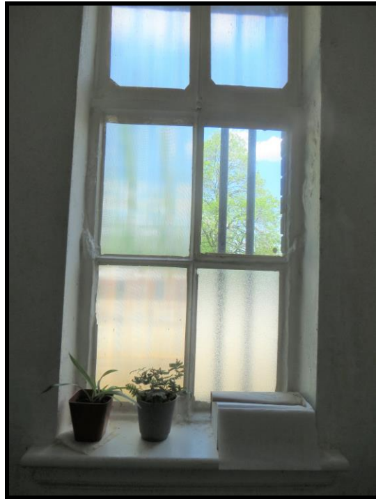
Image 29: Detail of Window in Rewind Room Washroom of 1014 King Street West, Hamilton – Westdale Theatre (Photo taken on May 29, 2017; Facing East)
