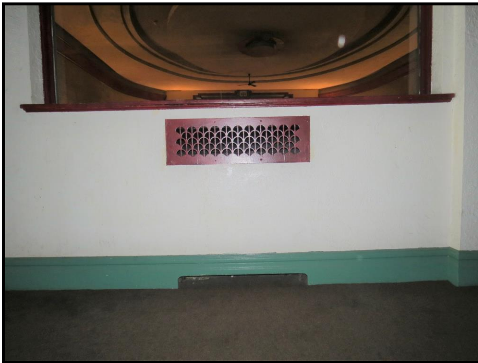
Image 36: Detail of Metal Grate under window to Auditorium of 1014 King Street West, Hamilton – Westdale Theatre (Photo taken on May 29, 2017; Facing West)
