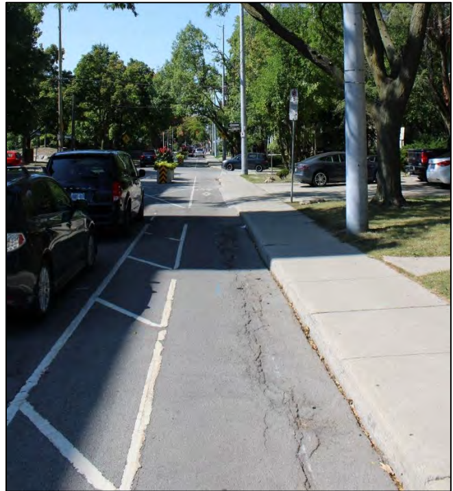
Herkimer Ave, Hamilton Parking protected bicycle lane as planned on Young St
