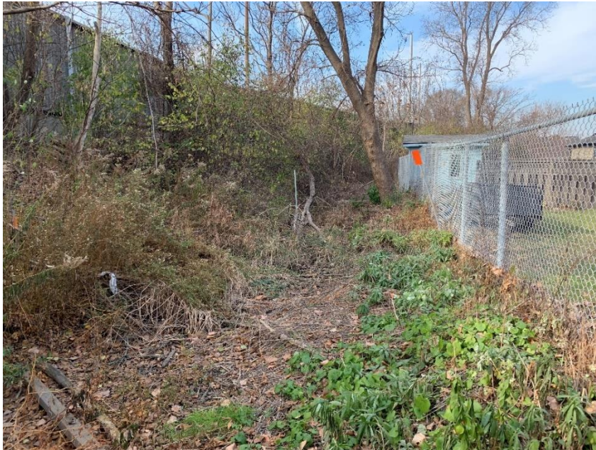
Plate 12: View storm sewer installation area and ditch rehabilitation at the western end of Fletcher Avenue (A.S.I., 2022).
