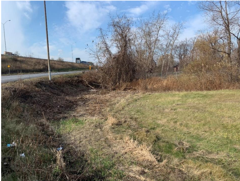
Plate 14: View of southern area for the storm sewer installation and ditch rehabilitation near the intersection of the on-ramp for the Queen Elizabeth Way and Beach Boulevard (A.S.I., 2022).
