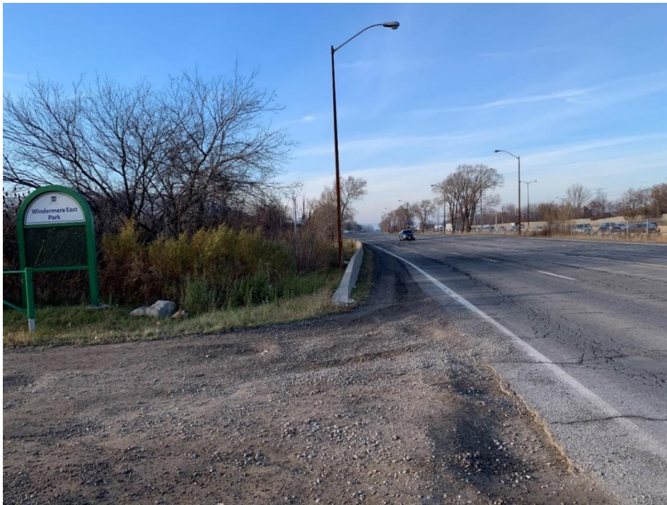
Image 14 Existing ditch rehabilitation between Eastport Drive and the Queen Elizabeth Way; Area is disturbed, no potential
